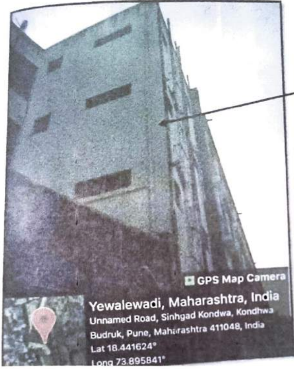
Photograph of Rain Water Harvesting Pipe from Terrace:
